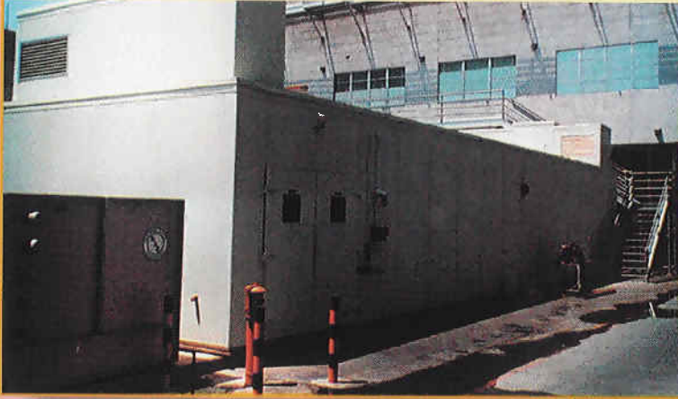
Acoustical enclosure with "single pass" silenced ventilation system.
