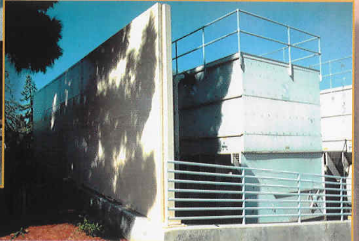
Soundwalls reduce community cooling tower noise.
